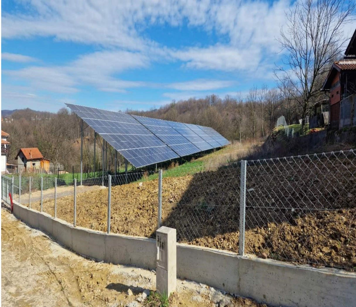
Figure 4. The solar power plant
